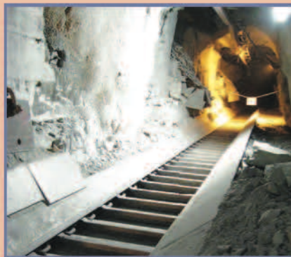
Cat Rock Flow System conveyor with drawpoint on left
